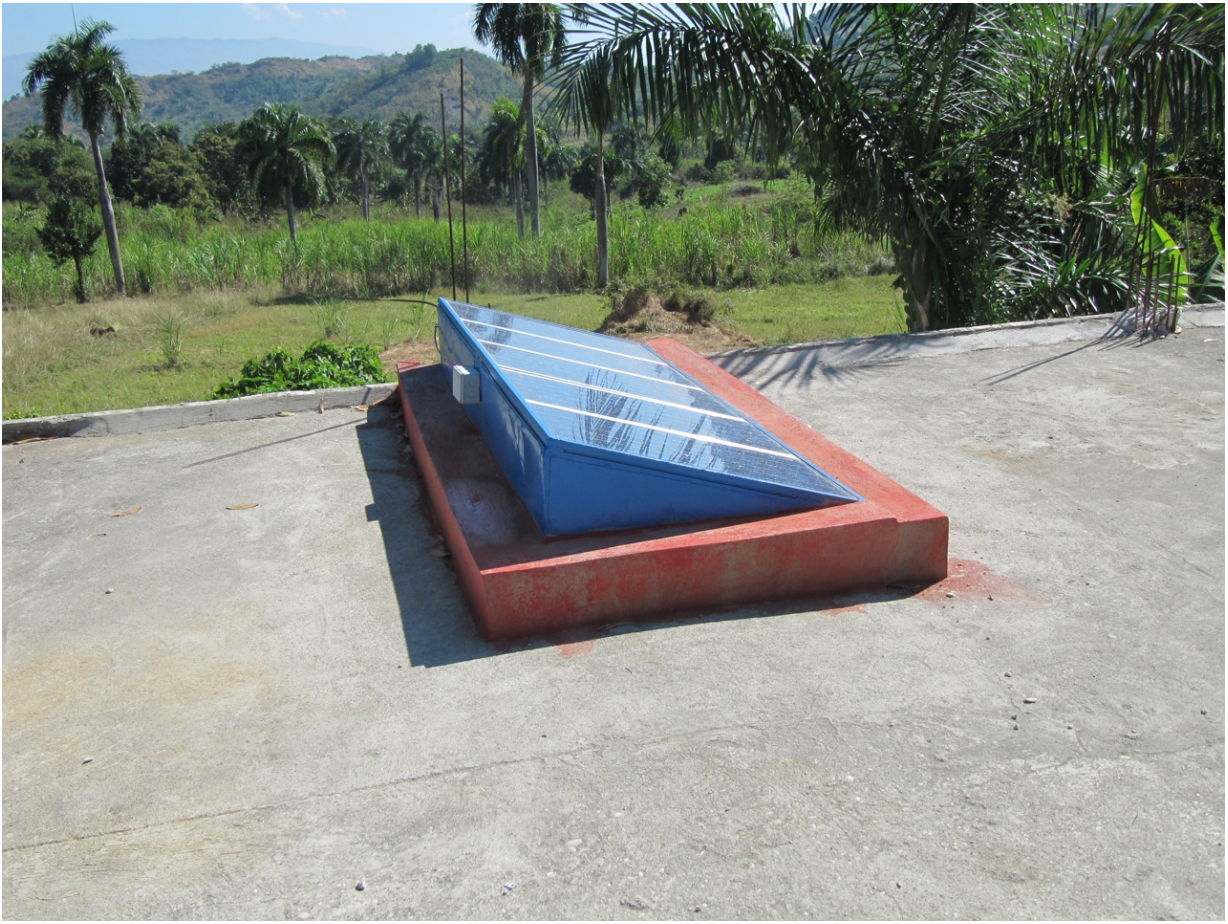
Figure 3: A well-protected PV array. Note that metal frame enclosures extend downward on the sides and are not easily removable from the top.
